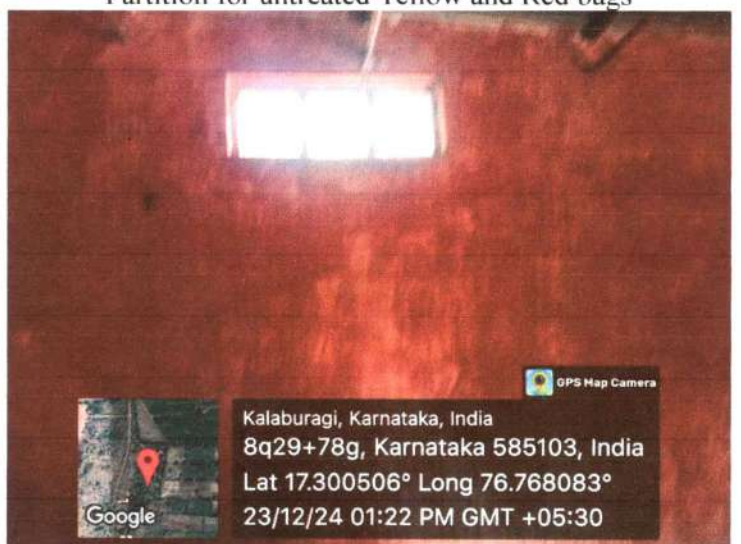
Ventilation for untreated storage room
