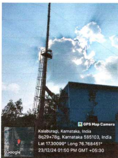
Stack with port hole and platform
