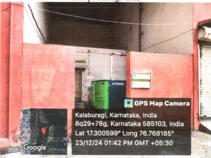
DG Set room
